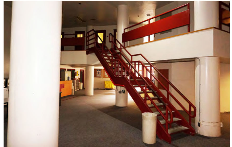
Figure 39: The typical housing unit is irregularly planned, with large structural concrete columns throughout, interfering with visual supervision.
